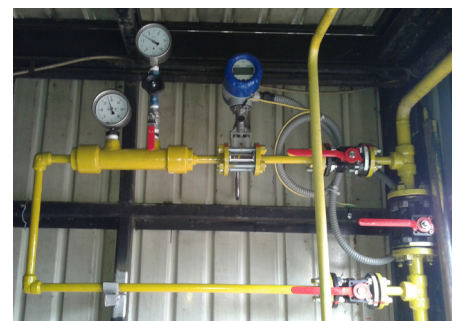
Vortex flowmeter mounted in a bypass line
